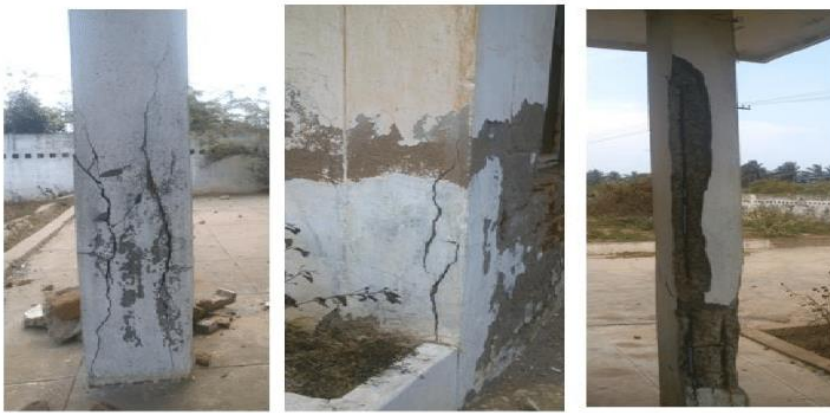
(Fig 4. Examples of cracks in concrete [8])
